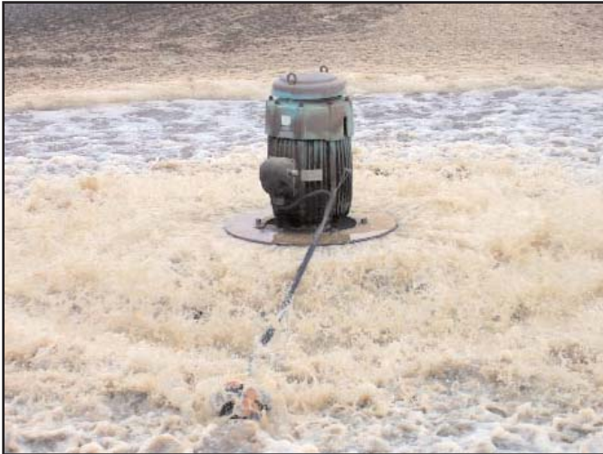
Close-up View of Clarifier
