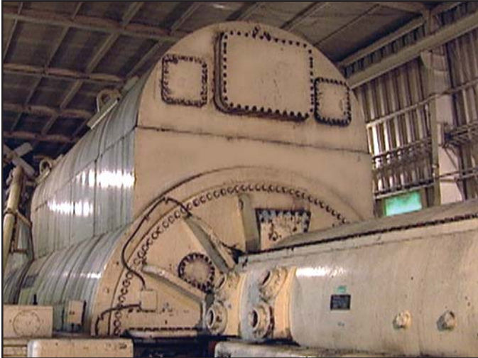
One of KCP&L's massive turbines used for power generation
