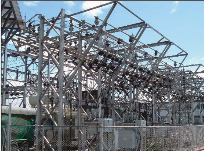
Substation La Uruca
