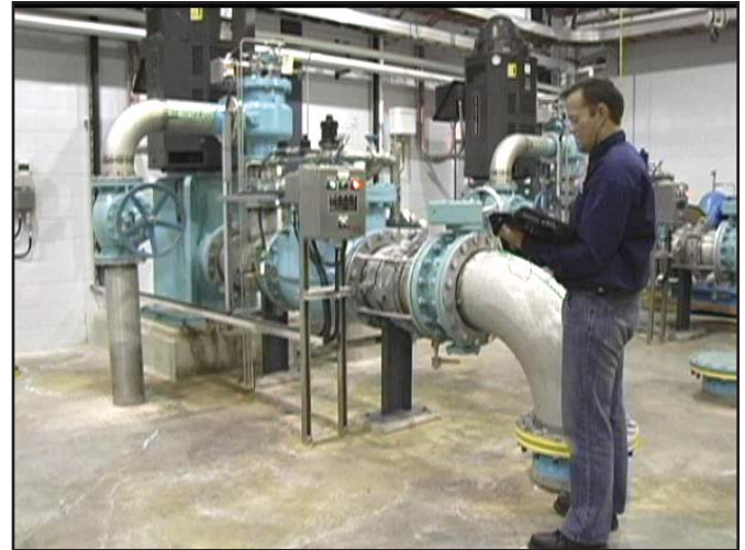
Operator utilizing tablet to turn on pump.
