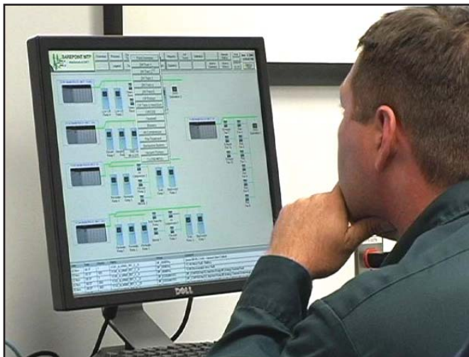
Operators can stay in the control room and monitor all plant processes and analytical equipment from there.
