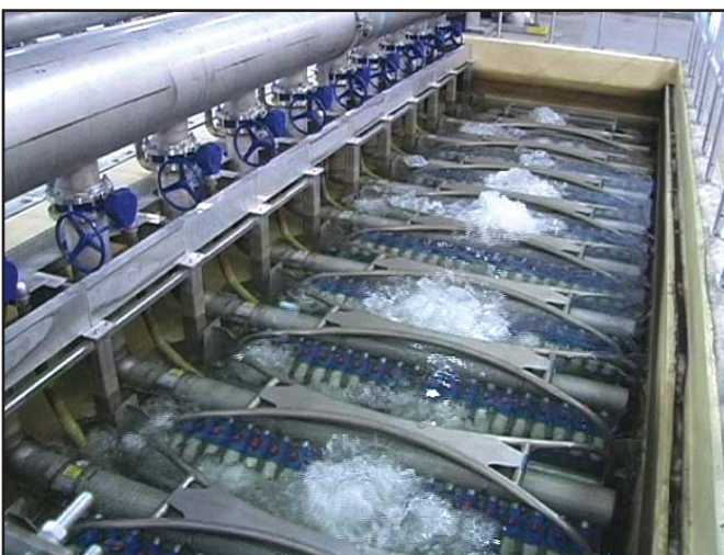
Backwash cycle on the Ultra Filtration trains.
