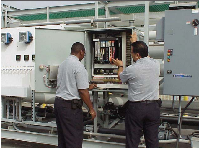
Workers at the LBWD Treatment Plant
