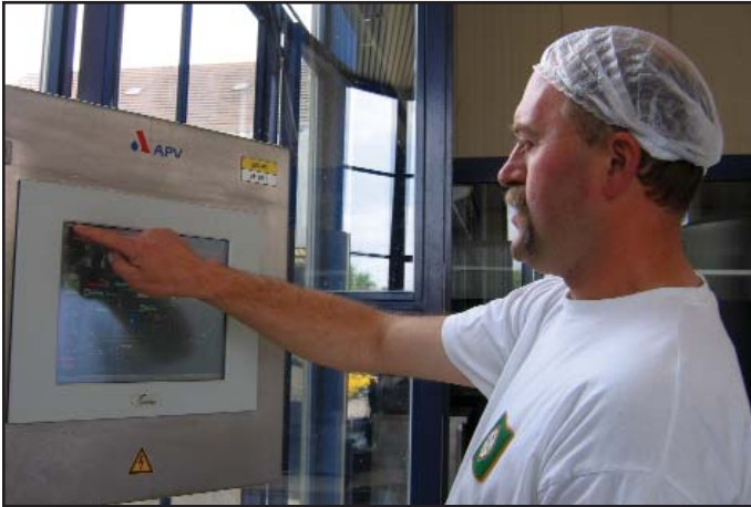
Operator on the plant floor using InTouch HMI Software
