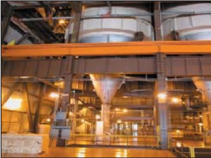
The incoming coal is fed into 1,000-ton hoppers before entering the coal pulverizers.
